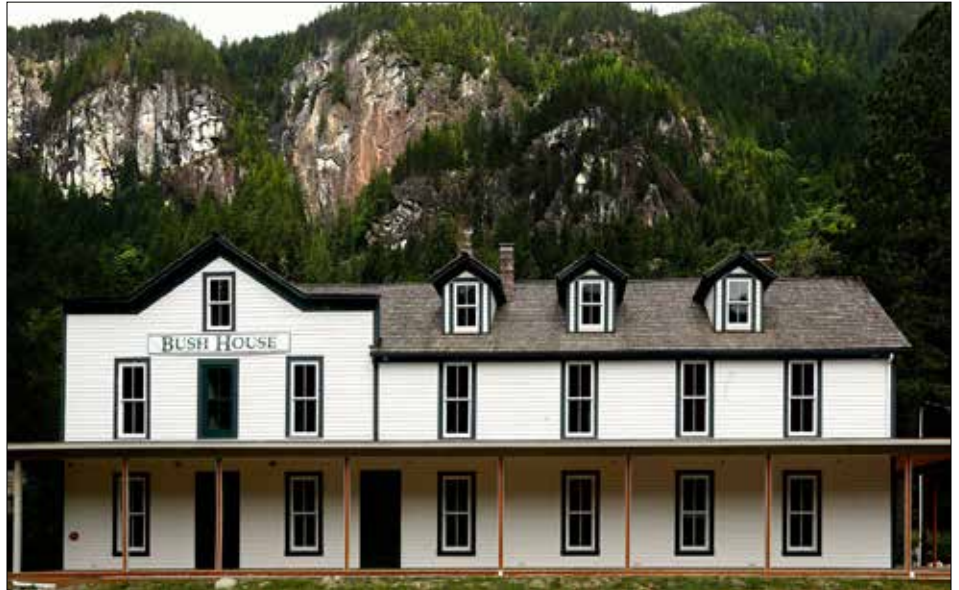
The Bush House rehabilitation in Index received a grant from the Valerie Sivinski Fund. Photo by Dan Bates, The Herald.
